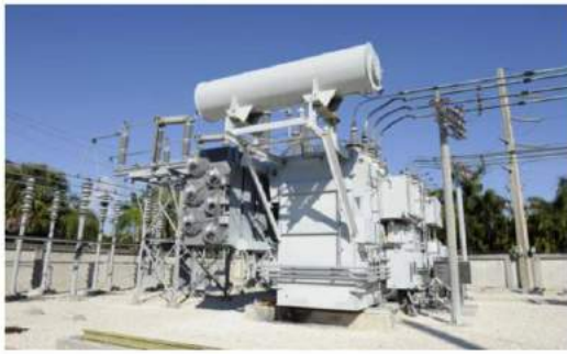
Smart devices have been installed on 78 substation transformer banks.
